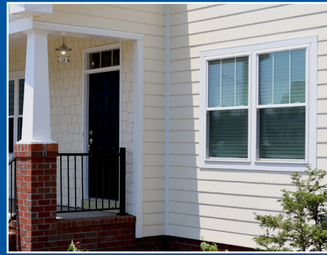
Two mullied double hung windows allow for more light to enter the home while minimizing visual obstruction and using less framing material during installation.
